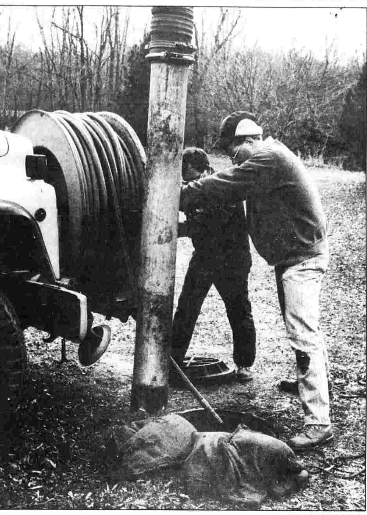
READY FOR WATER — Tony D'Amato, left, and Fred Lea, both of the Manchester Sewer Division, clear a bypass pipe for water flow to the skating area at Charter Oak Park.
